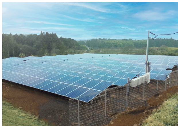
Kasama City Solar panels [Ibaraki]
