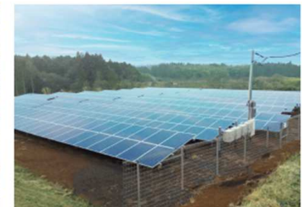
Kasama City Solar panels [Ibaraki]
